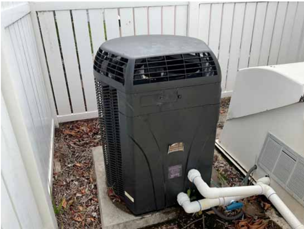
Pool Equipment, Heater
